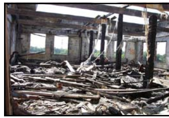
Figure 3 - Mill Building Fire Destruction courtesy of Michael Malinowski, AIA
