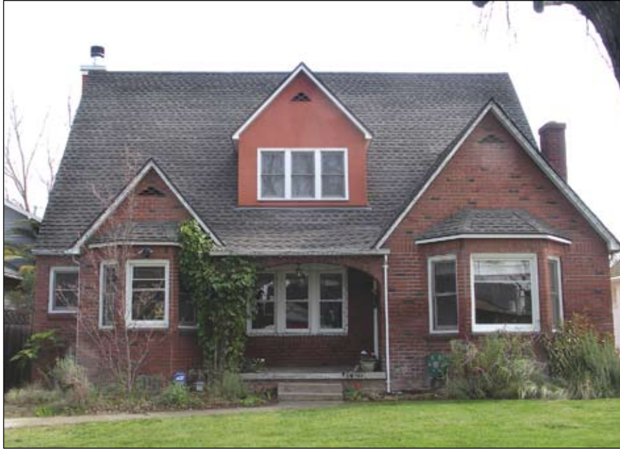
Mills Builders added a second floor to this home and a casita in the back
